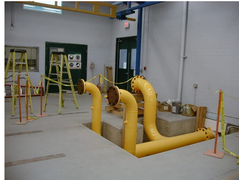
Indoor Piping to Reference Meters and Test Meters
