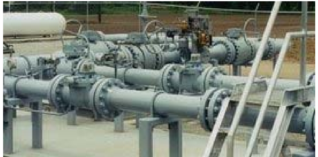
But some installation problems are not so apparent
