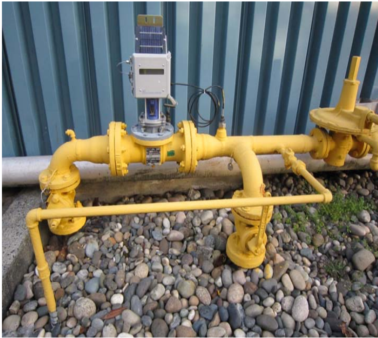
Some installation problems are obvious
