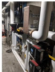
Existing HX and Pumps
