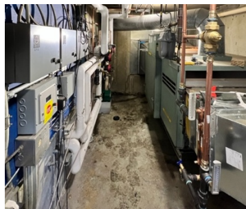
Existing Makeup Air Unit
