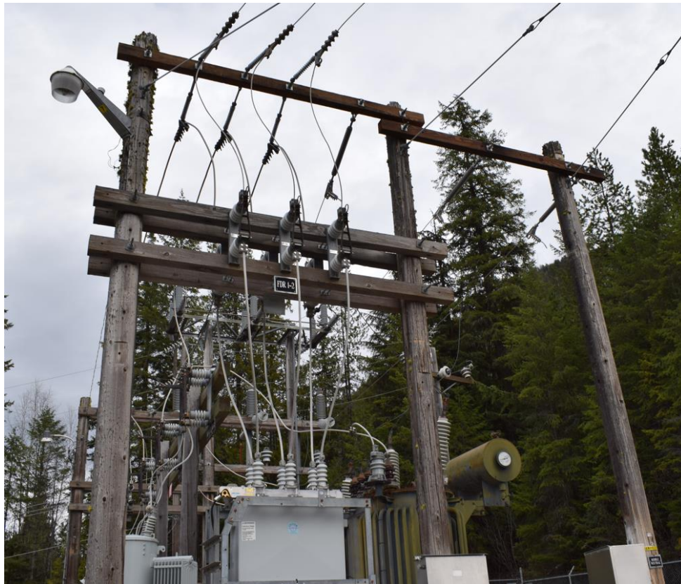
Figure 3-9: Wood Pole Condition at the Existing Hearn Substation
